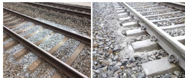
Figure 1. White spots of ballast breakdown (left) (Sysyn, et al. 2020) and Mud pumping induced by ballast fouling (right) (Nurmikolu et. Al (2013)
