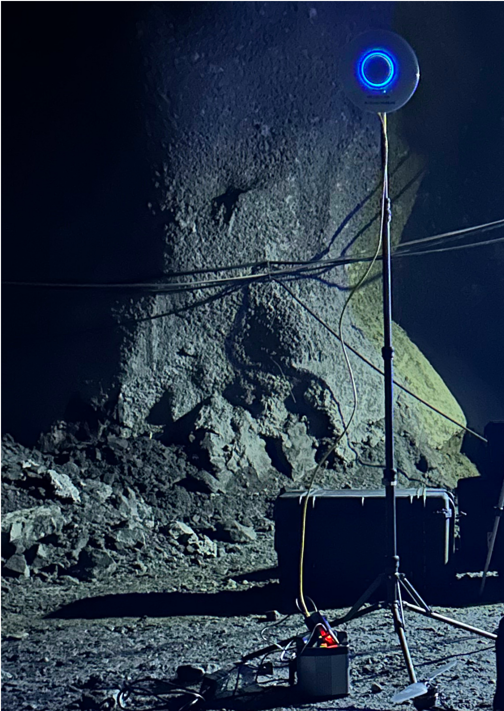
Fig. 13: One of the nodes in the mobile Wi-Fi mesh used to provide communication for the task coordination. The Ubiquiti U6 Pro is mounted on a tripod and connected to a battery to allow for easy and quick deployment in the underground environment.
