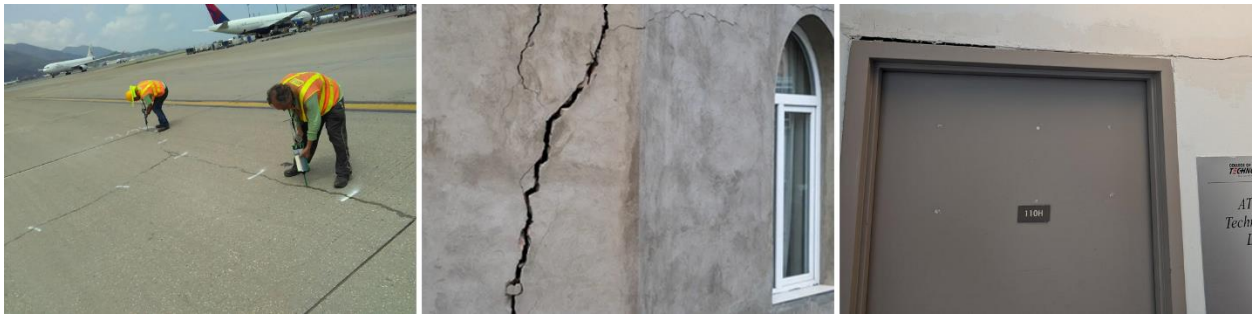
Fig. 1. Surface cracks in different environments: an airport runway under repair (left), a building wall post-earthquake (middle), and a crack above a door (right).
