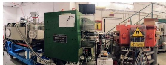
Figure 13 PADME experiment installed in BTF1 bent line.
