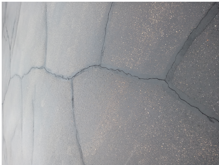
Figure 4: A system of cracks in a parking lot
