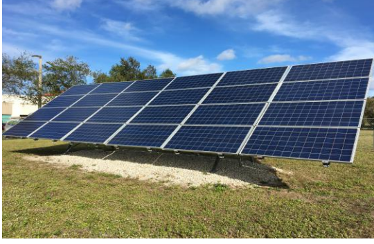
Fig. 1. Photovoltaic unit installed at FAU Boca campus
