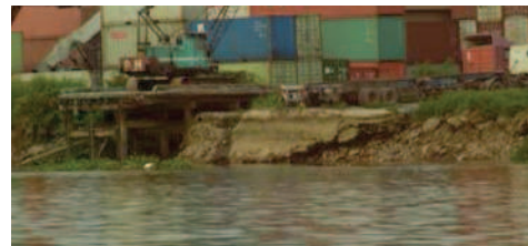
Figure 1 Riverbank failure along Saigon River
